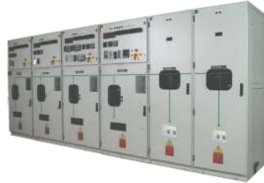
11 KV HT Panel
