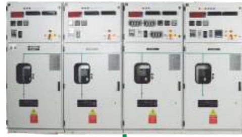
33 KV HT Panel
